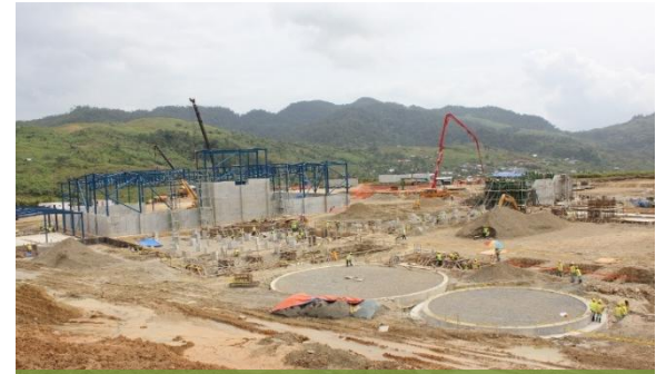
Plant site overview
