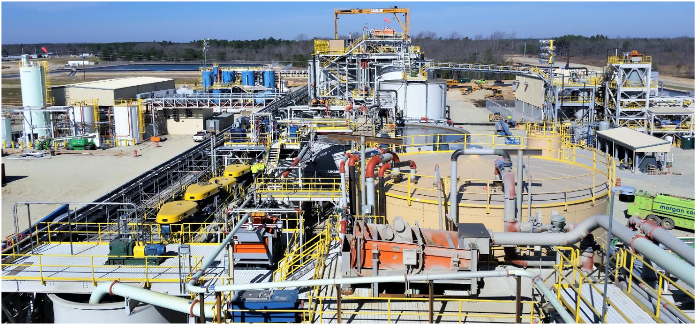
Figure 3 – Process Plant Overview
